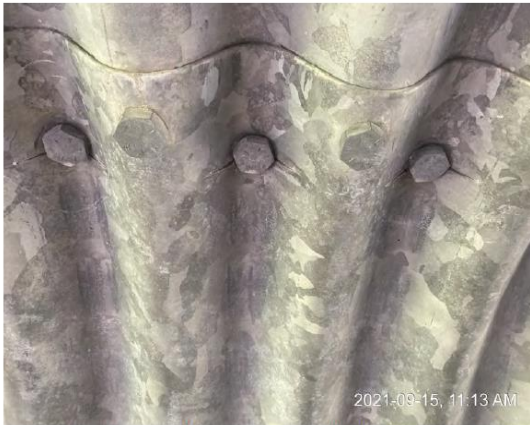
Image 6 – Horizontal shear cracks along north bolt line (looking north)
